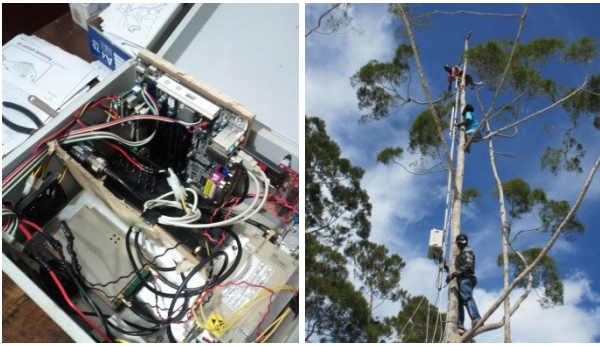
Figure 2: Our Base Station and its installation.
