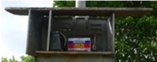
Figure 3: Battery of a villager being charged by the community-owned solar panel
